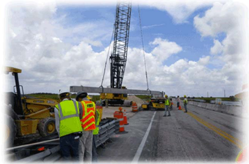
The first of 34 test piles is installed for the Tamiami Trail bridge project.
